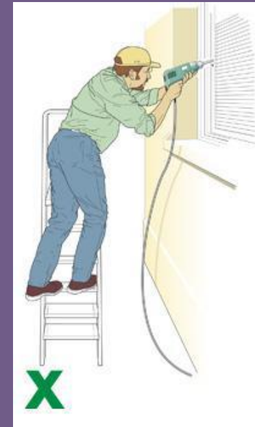
Incorrect - steps side-on to work activity
